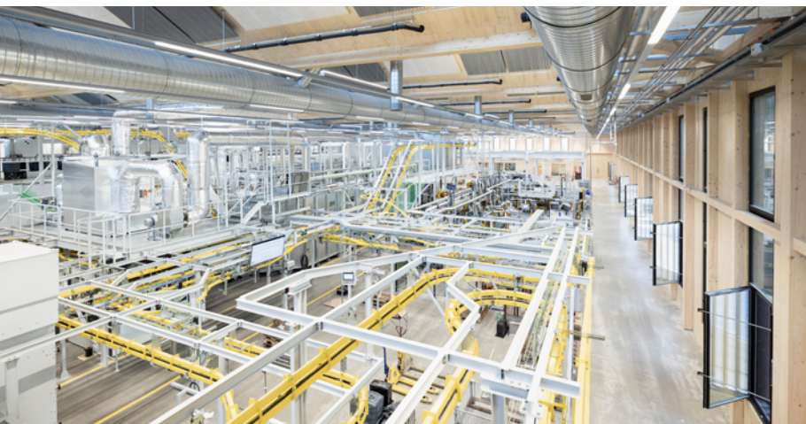
V-ZUG production facility with enamelling plant (high-temperature process) for ovens
